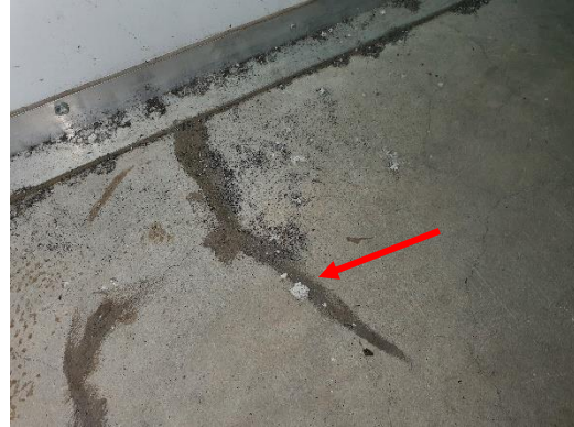
Image 4: Return Air Room - Vermiculite debris
