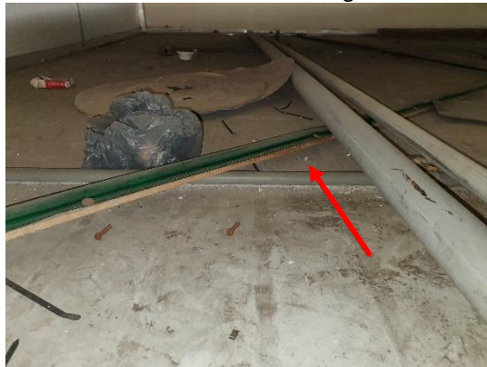
Image 5: 5 th Floor Main Room - Vermiculite debris on top of North Plant
