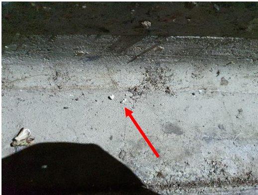
Image 1: Filter Room - Vermiculite debris
