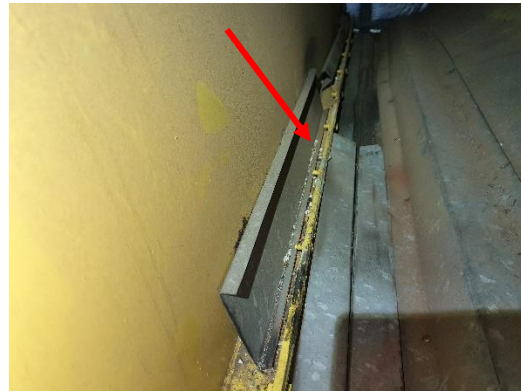
Image 2: Filter Room - Vermiculite debris
